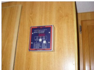
A Tri Metric 2020 battery monitor system.
